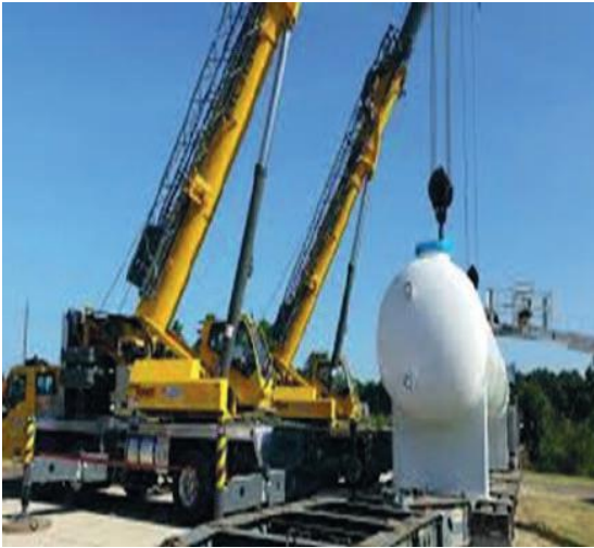
Lift and Rope of Lift
